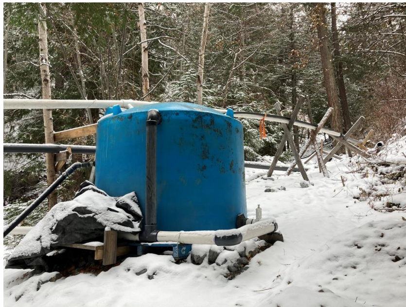
Overland piping and emergency storage tank at a small water system after a debris flow caused by an atmospheric river severely damages the system in 2021.
