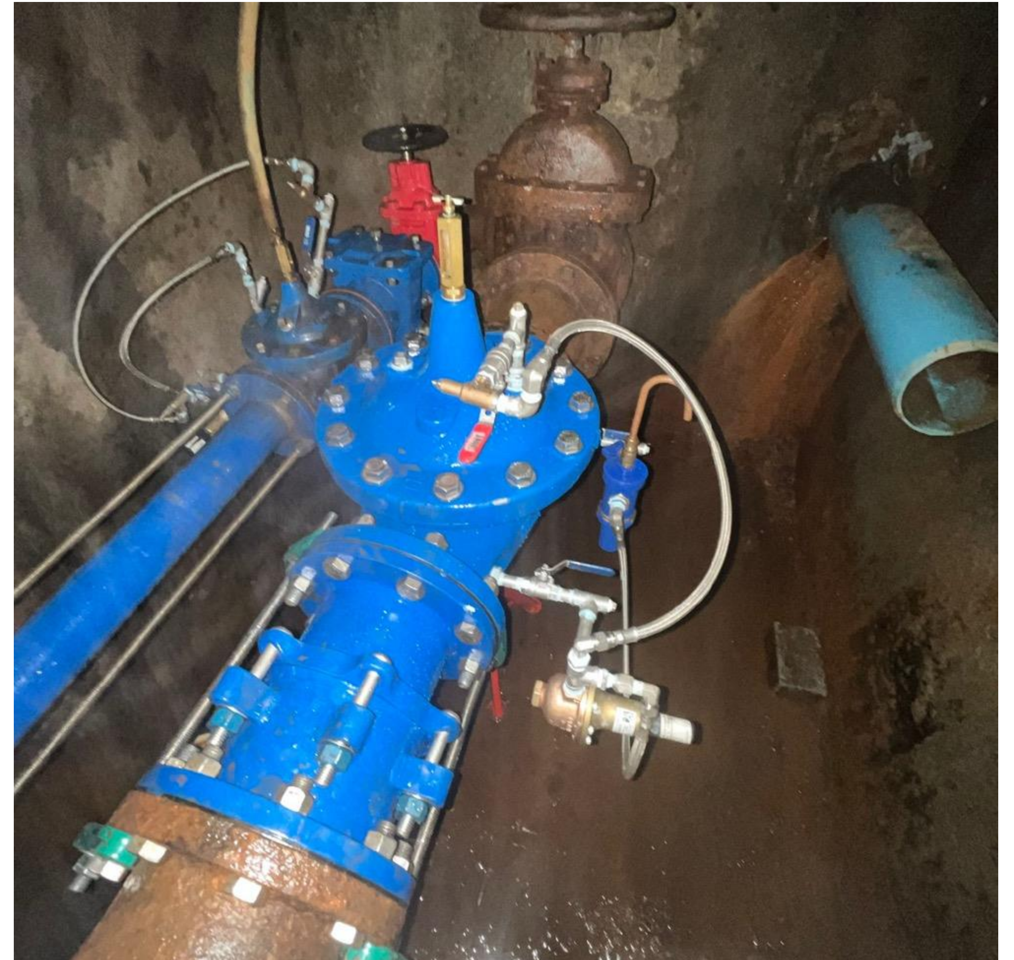
Newly installed upgraded PRV's
