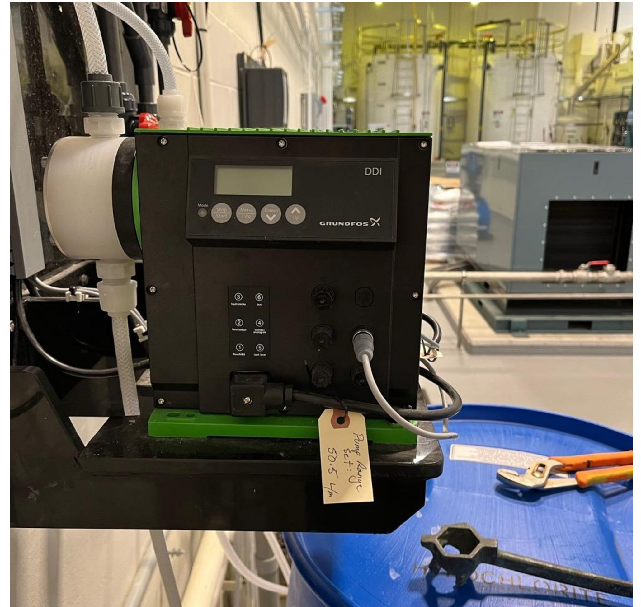
Back up dosing skid. Two Grundfos pumps with two 12% Hypochlor barrels.
