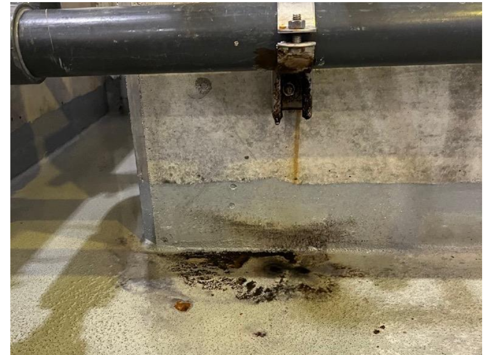
Leak underside of this bracket.
