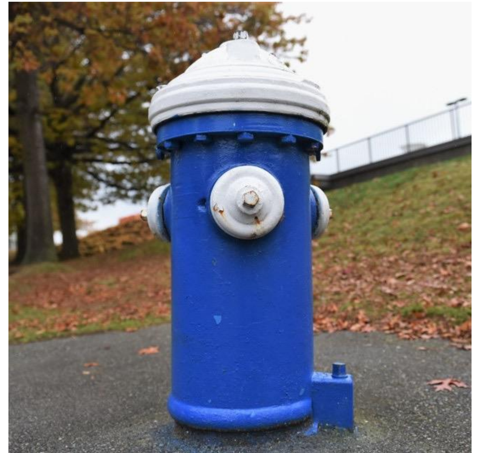
DFPS hydrant Vancouver BC. Photo by Brenden Kergen-Vancouver is awesome.
