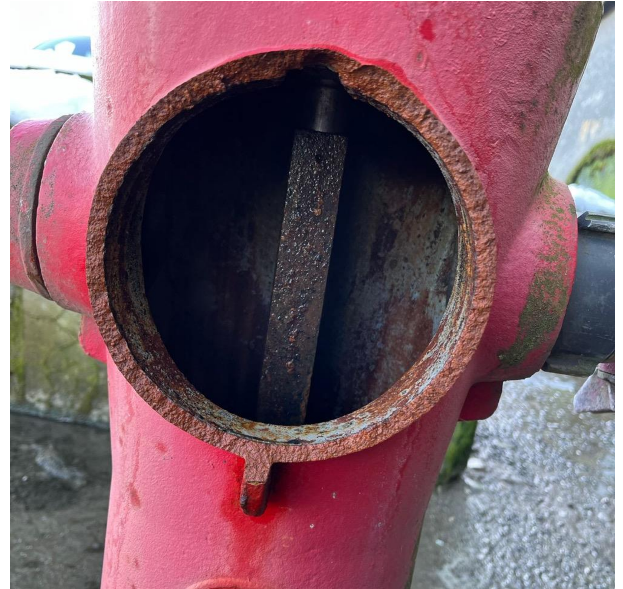
Hydrant left on during freezing temperatures.
