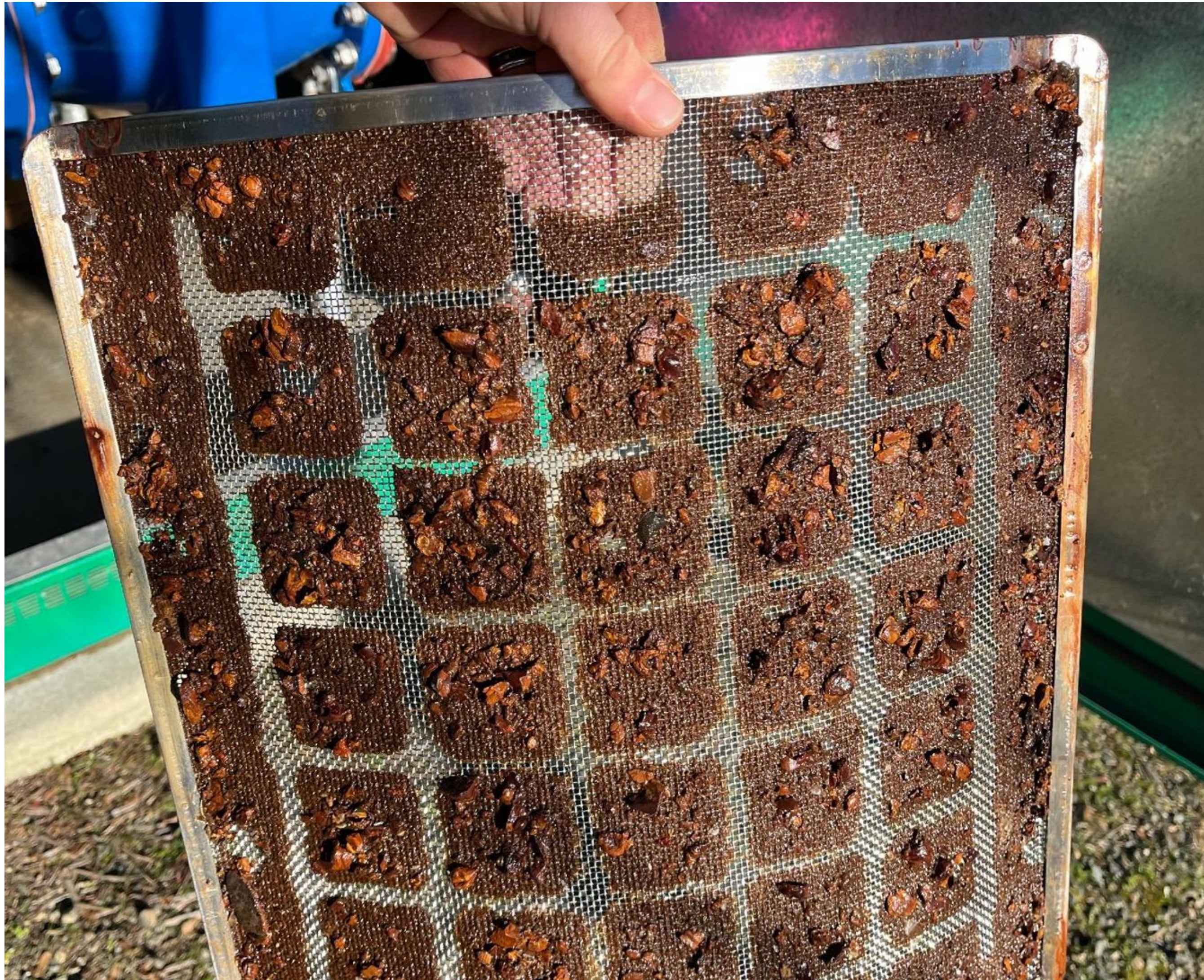
Bi-Annual PRV screen cleaning. This valve had seen high flows do to main breaks and a sustained fire hydrant port blow out.
