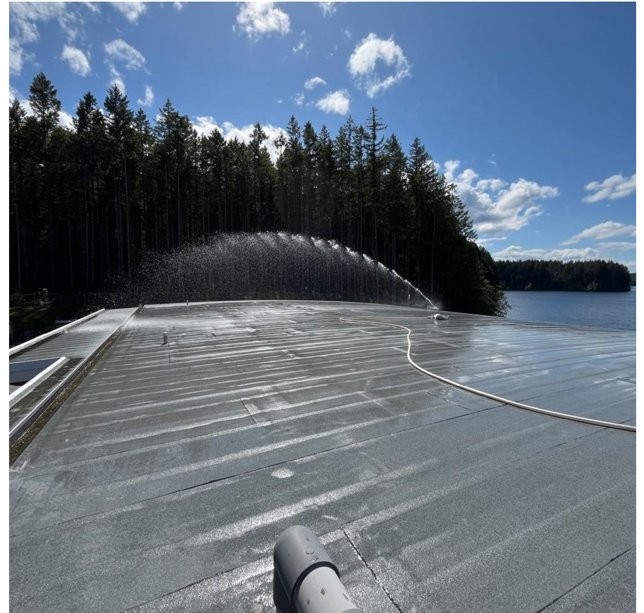
Fire Bozz Mini sprinkler being deployed for summer months. Part of our effort to protect critical infrastructure from the potential threat of wildfire.
