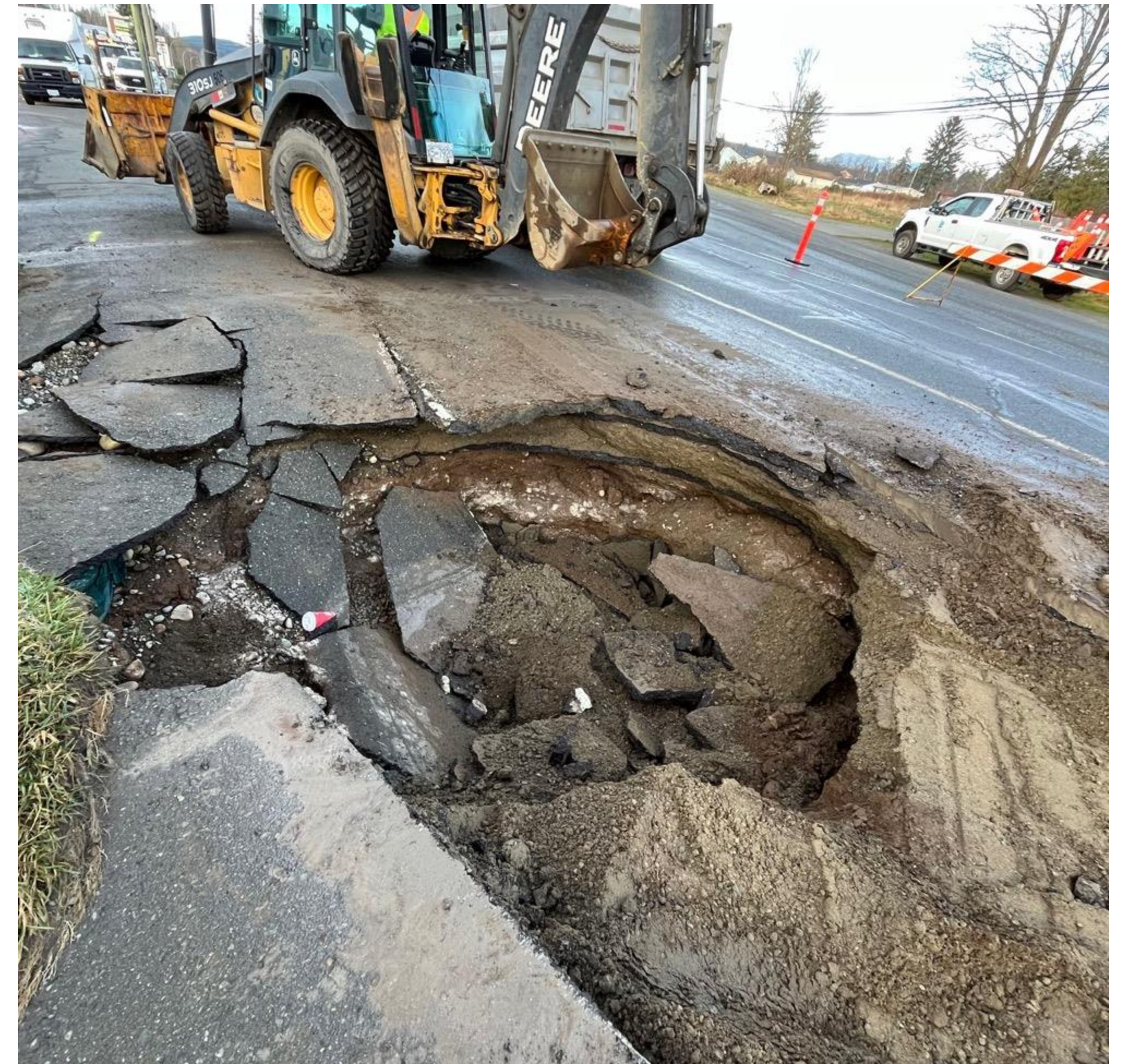
200 mm Cast Iron water main popped.
