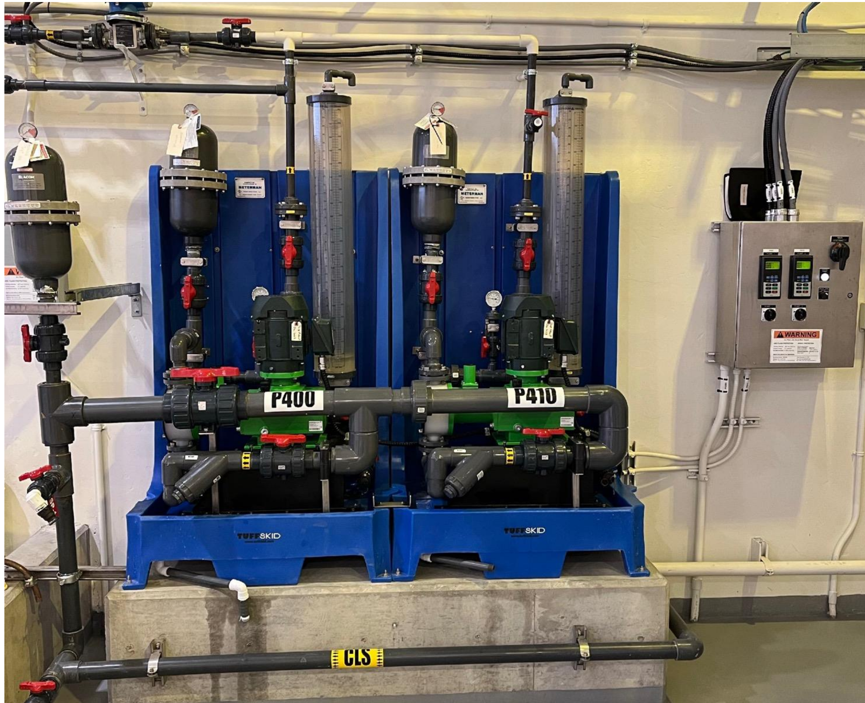
Main dosing pump skid. Bottom 2" line left bracket rubbed a small hole do to vibration.
