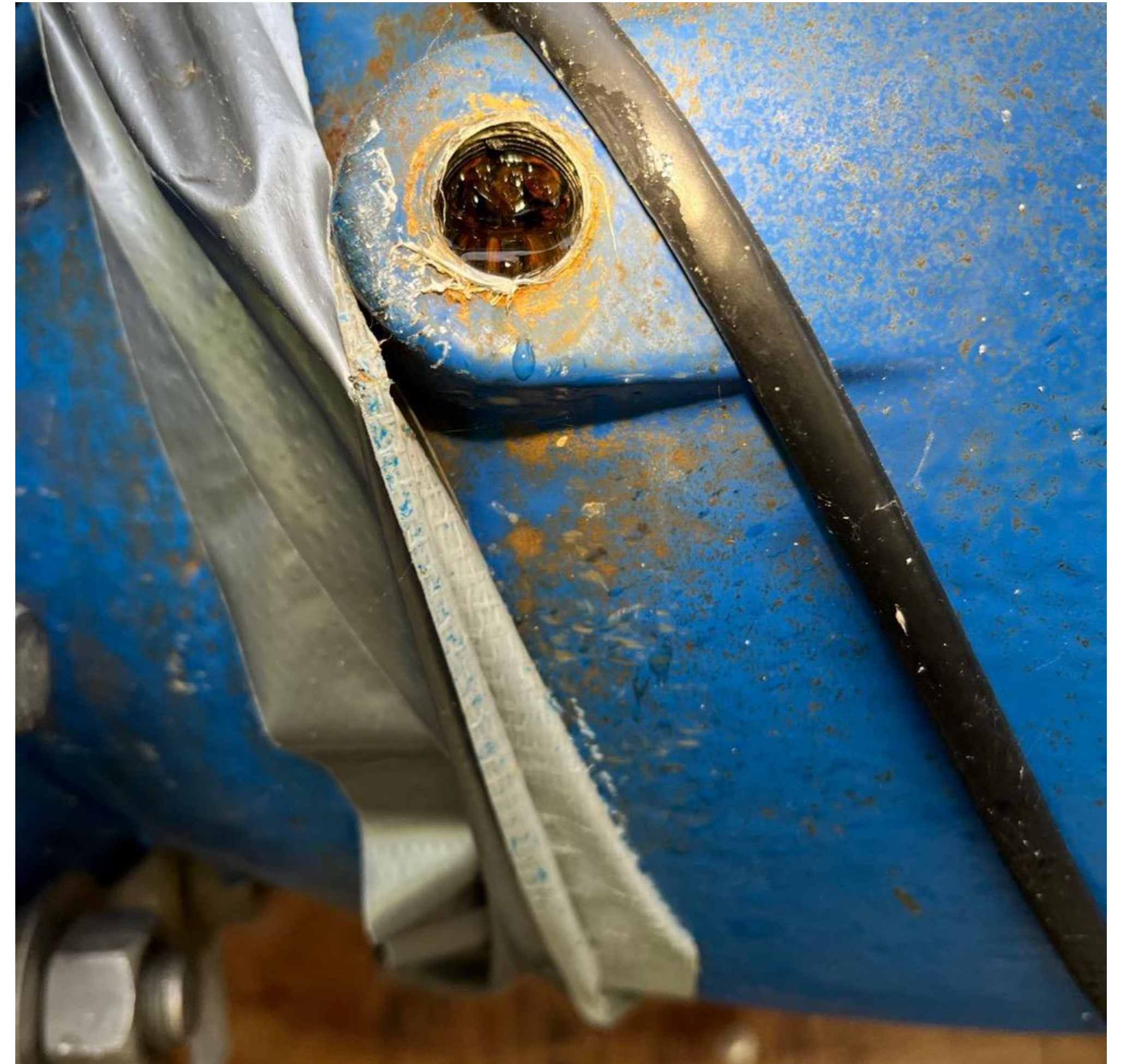
Plugged port on an unlisted valve. Showing the importance of P.M. schedules.
