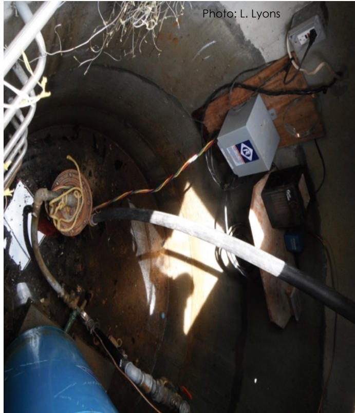
Drilled Well in a Pit or Vault
